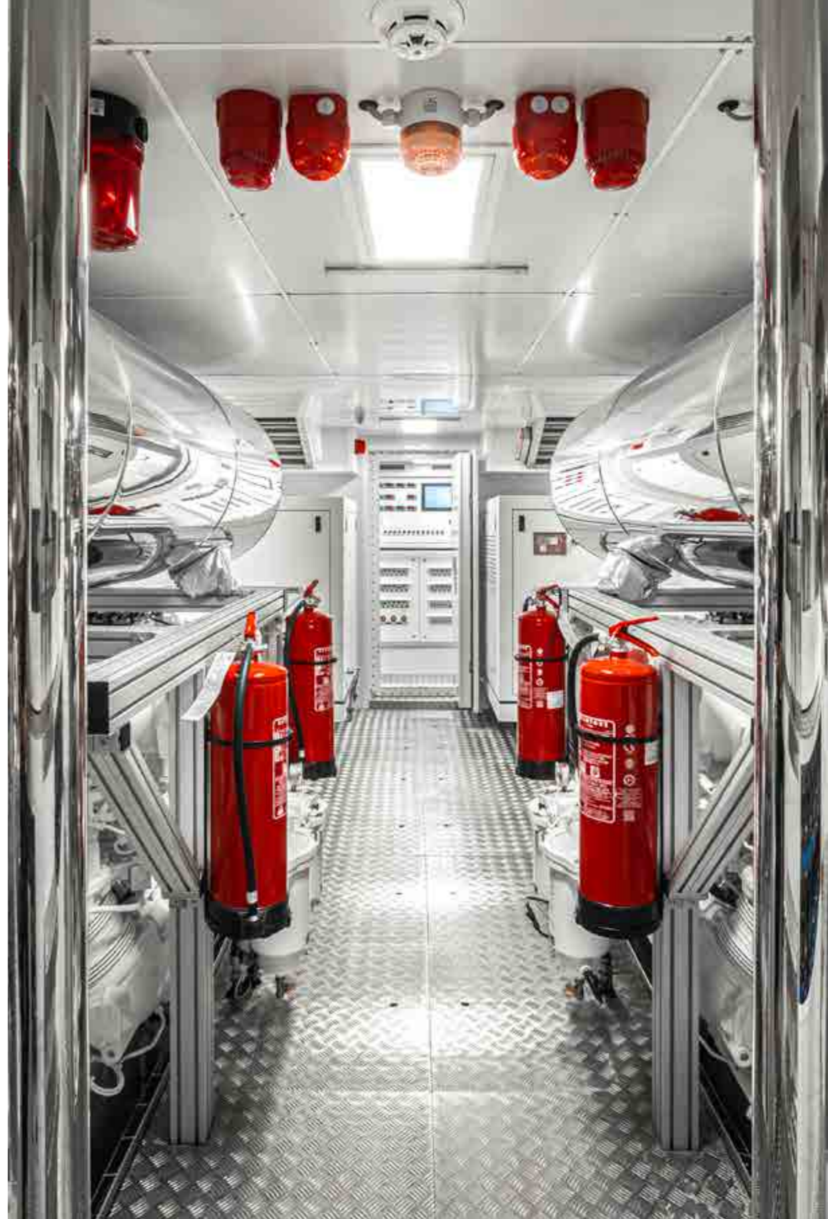
LOWER DECK | ENGINE ROOM
